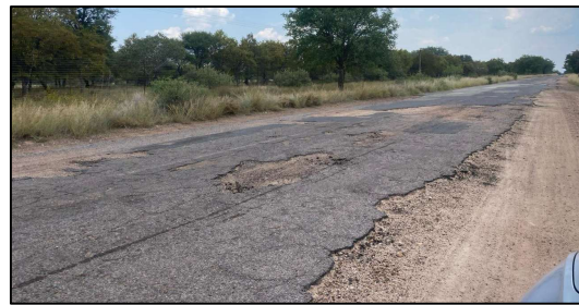
D2460 Road Condition – Paved (Extremely Poor))
