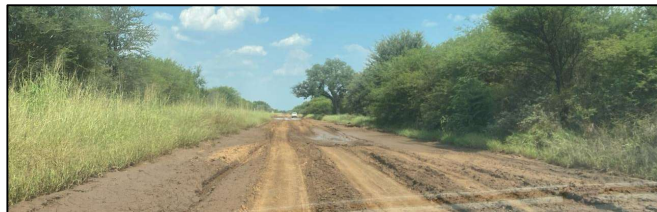
D1309 Road Condition – Gravel (Poor)
