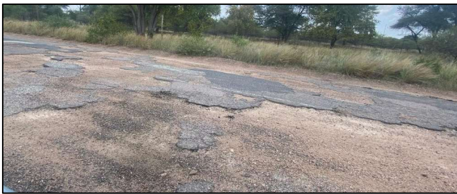
D2460 Road Condition – Paved (Extremely Poor)
