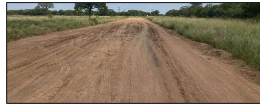
Road D1309 Condition – Gravel (Poor)
